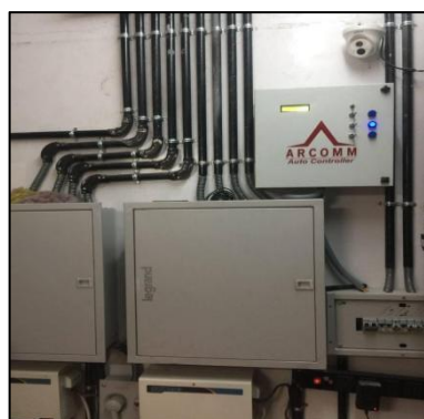
Auto Controller deployed in SBI ATM
