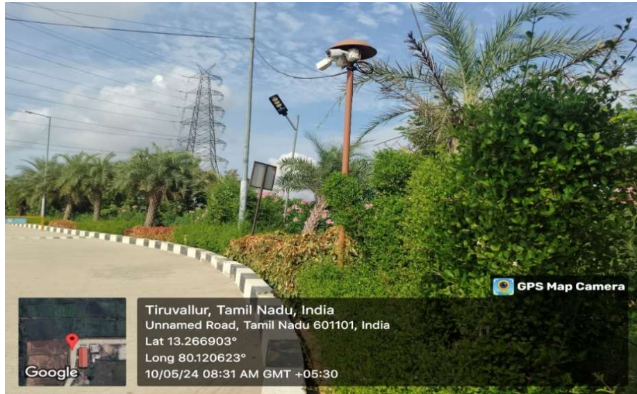
CCTV installed for campus surveillance
