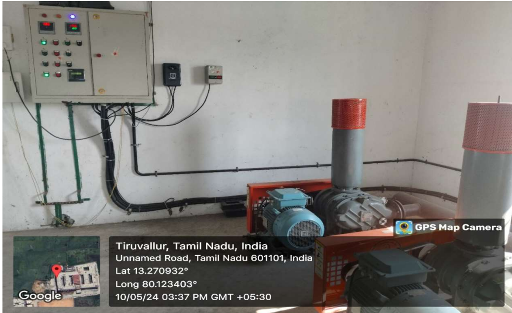
Equalization Tank in Liquid Waste Management Plant at Medical Campus
