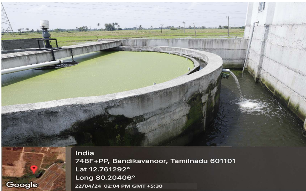
Processed Water Collection Tank in Liquid Waste Management System at Medical Campus
