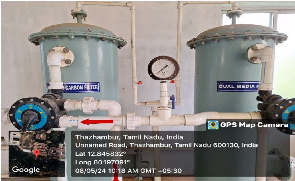
Filtration Units in Liquid Waste Management System at Thazhambur Campus
