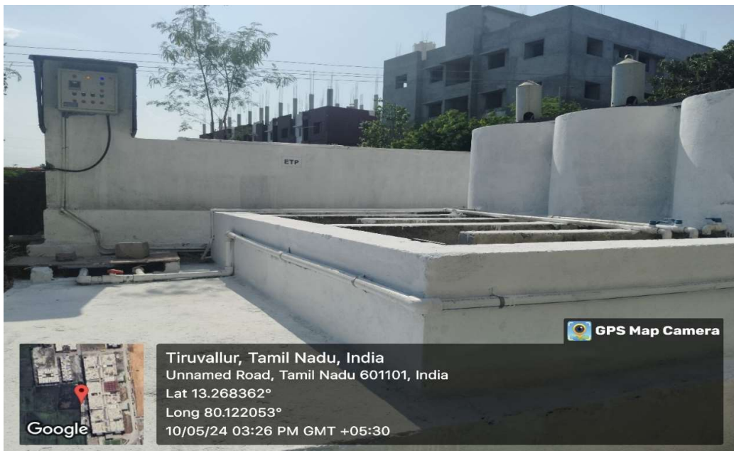
Liquid Waste Management Plant at Medical Can
